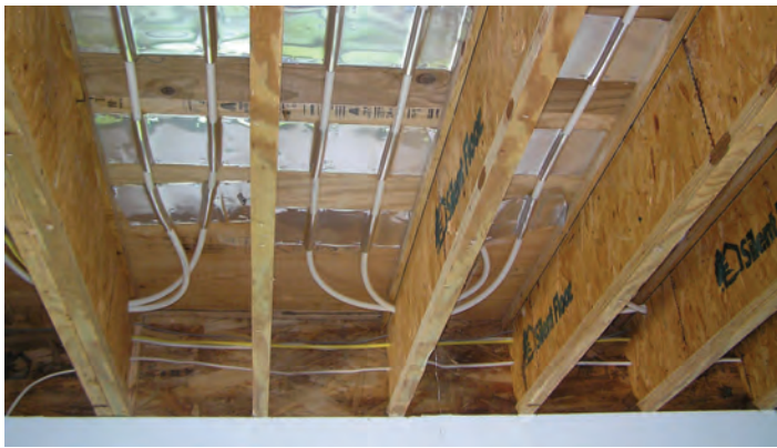
Radiant floor systems are relatively easy to install in buildings with unfinished basements offering easy access to the underside of the main-level floor.
